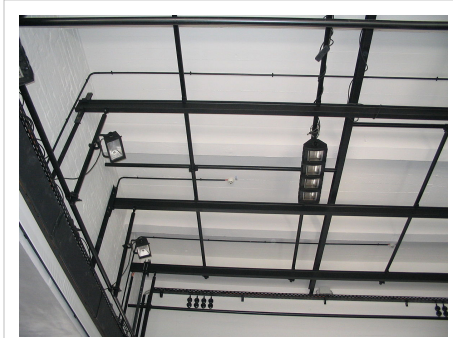
Ceiling with light fixtures for stage in the Festsaal
