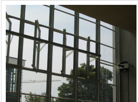
Mechanically opened windows
